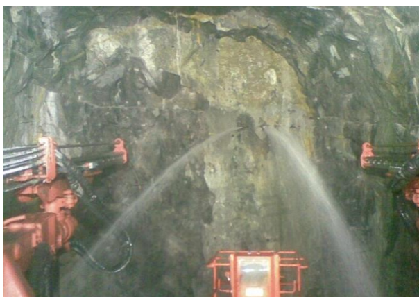
Fig 4 Water ingress along sub-horizontal joints
