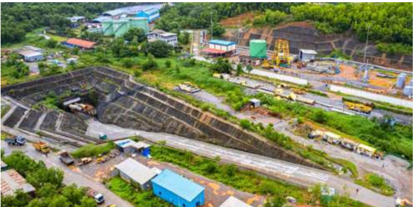
LPG cavern at Mangalore, Karnataka
