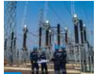
Utility & Offsite facilities, including Captive Power Plants
