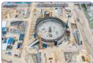
NHT-CCR Reforming Unit at Arzew Refinery
