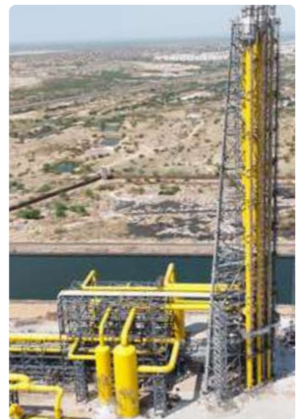
Demountable Flare System at HRRL
