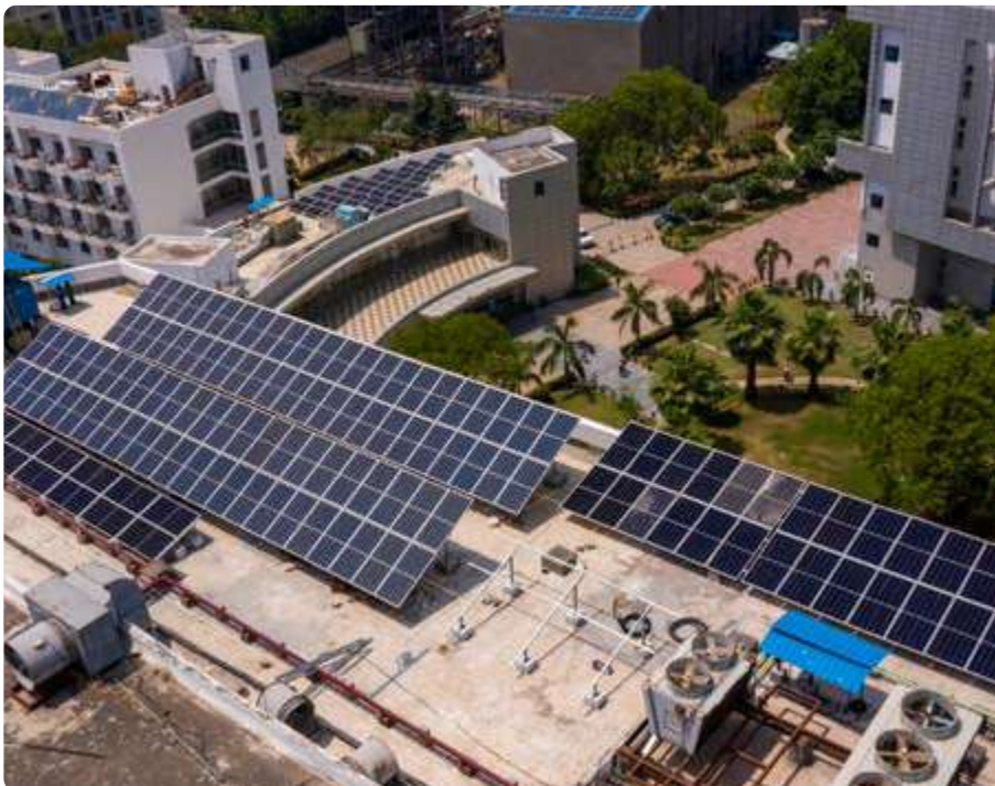
Rooftop SPV system at EIL Gurugram Office Complex
