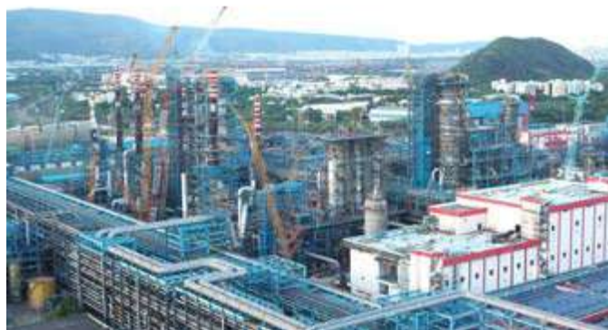
Residue Upgradation Unit (RUF) at VRMP
