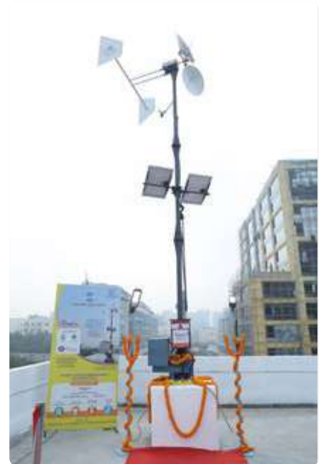
Low Wind Velocity Turbine installed at EIL Complex, Gurugram
