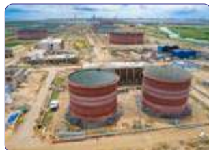
Crude Oil Terminal (COT) at Paradip, Paradip Numaligarh Crude Oil Pipeline (PNCPL)
