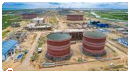
Crude Oil Terminal (COT) at Paradip, Paradip Numaligarh Crude Oil Pipeline (PNCPL) and NRL Siliguri Product Pipeline (NSPPL)
