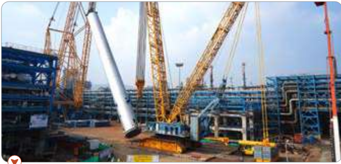
Vizag Refinery Modernization Project of HPCL, including India's first Residual Upgradation Facility (RUF) unit.
