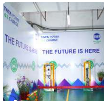
EV Charging Station at EIL New Delhi and Gurugram Complex
