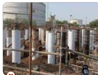
Onshore storage tank farm and associated facilities at GCPL
