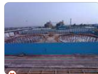
De-Bottlenecking and Augmentation of Cryogenic Facilities - LPG Import Terminal
