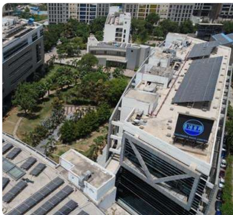
Solar PV system at EIL Gurugram Complex
