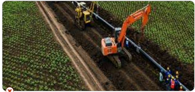
Krishnapatnam-Hyderabad Multiproduct Pipeline (425 km), commissioned
