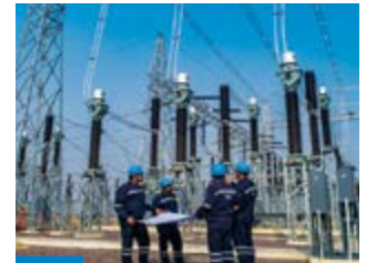
Utility & Offsite facilities, including Captive Power Plants
